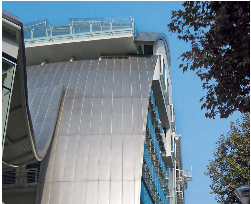
Rainfall has a natural cleaning effect in parts of the building envelope which are exposed to the elements. Photo: Centro Inox, Milan (I)
